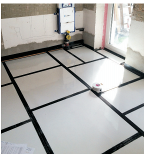
Internal floor insulation
