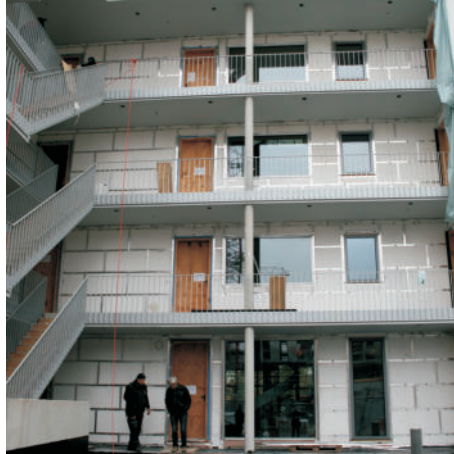
Installed QASA B1 area in Munich, Ackermannbogen Architect Werle
