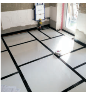
Internal floor insulation
